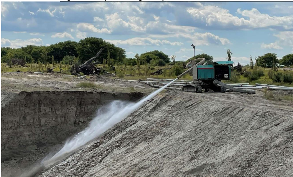
Semi-autonomous track mounted hydro-mining mining unit, top-down mining method Source: Fraser Alexander, SVM
